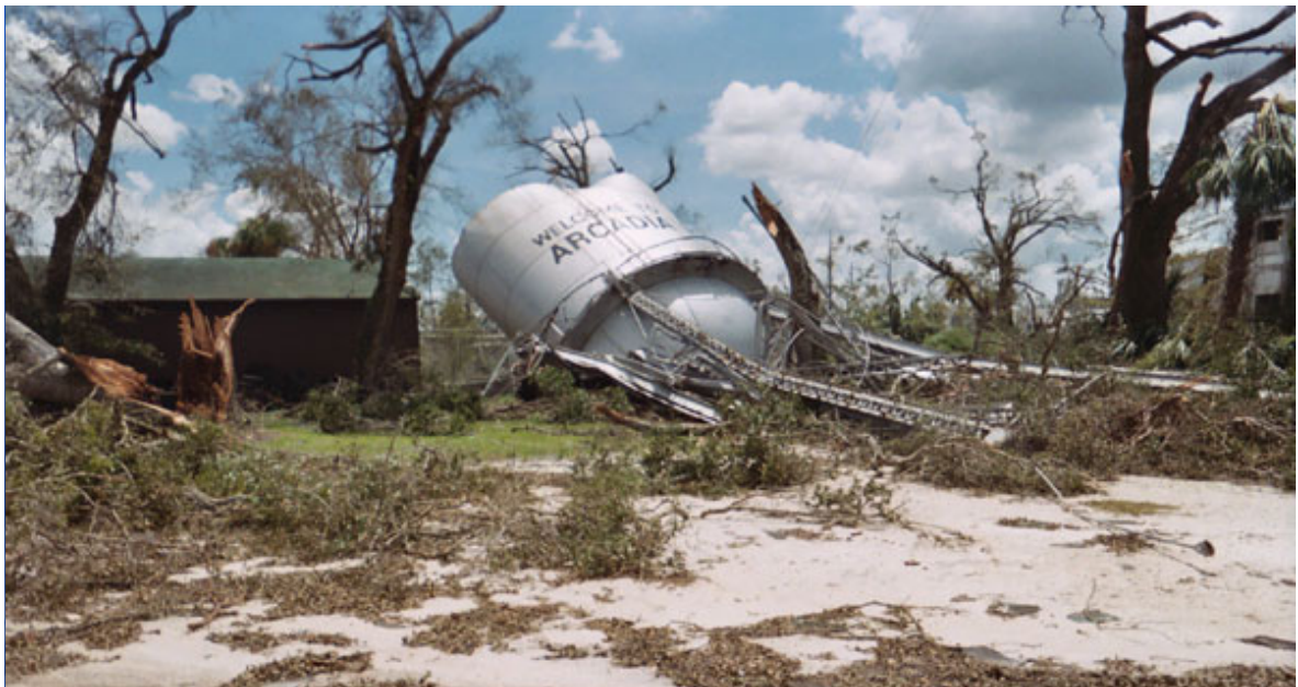
Storm damage from Hurricane Charley in Arcadia, © USGS
